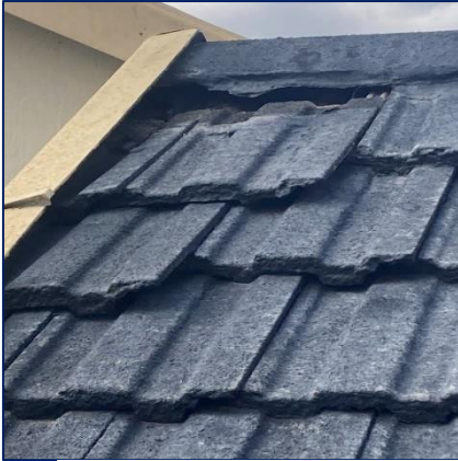
Figure 57: Loose Roof Tile
