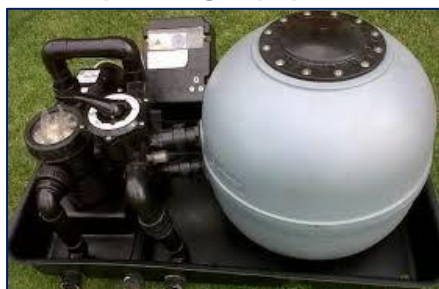
Figure 75: Pool Pump & Filter
