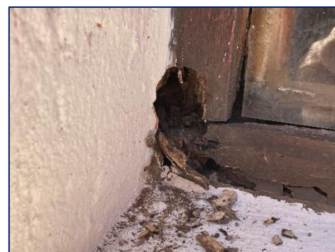
Figure 64: Water Damaged Window Frame
